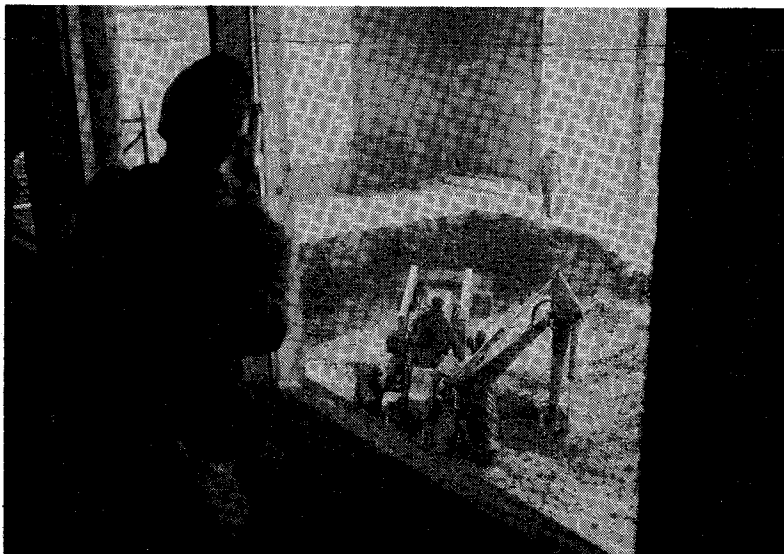
The new lodge addition continues to take shape. Presently, it is projected for service in December. Ultimately, the new adjunct will house expanded kitchen facilities, indoor/outdoor pool, men's lounge, pool lounge, locker rooms, and dining facilities.
